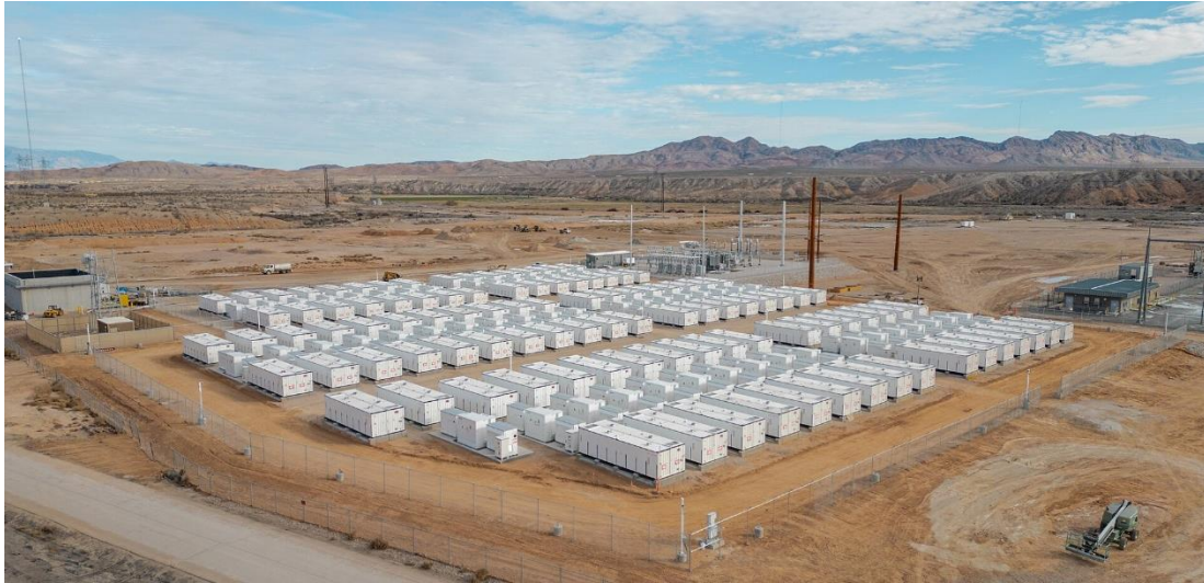
Fig. 1. An example of a large-scale battery energy storage system (BESS)
